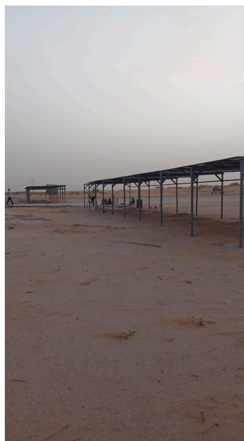
La structure photovoltaïque
